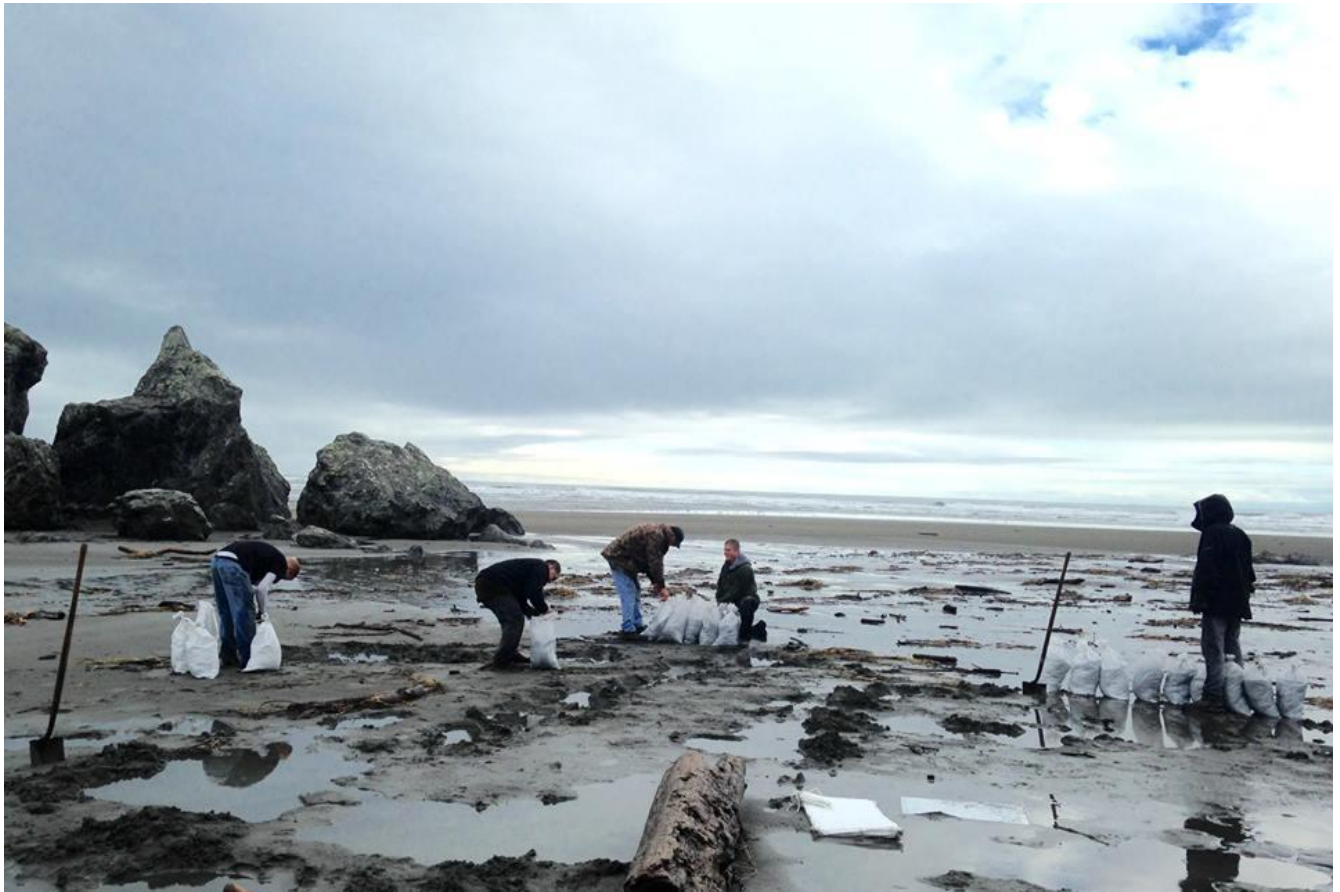
Above: Filling sandbags to shore-up the parking area after 2015 storms & high tides took their toll.
